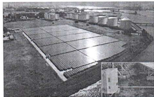
JTC Solar Farm, Singapore 5MW
